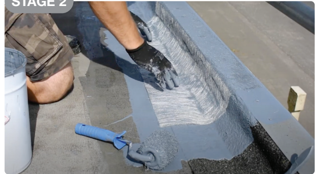
Reinforcement of the perimeter and construction details with STARFLEX liquid membrane and STARTEX NW DETAILS fabric.
